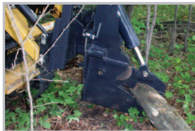
Fell trees can be sectioned for easy removal or clipped to length for firewood or compact loading.
